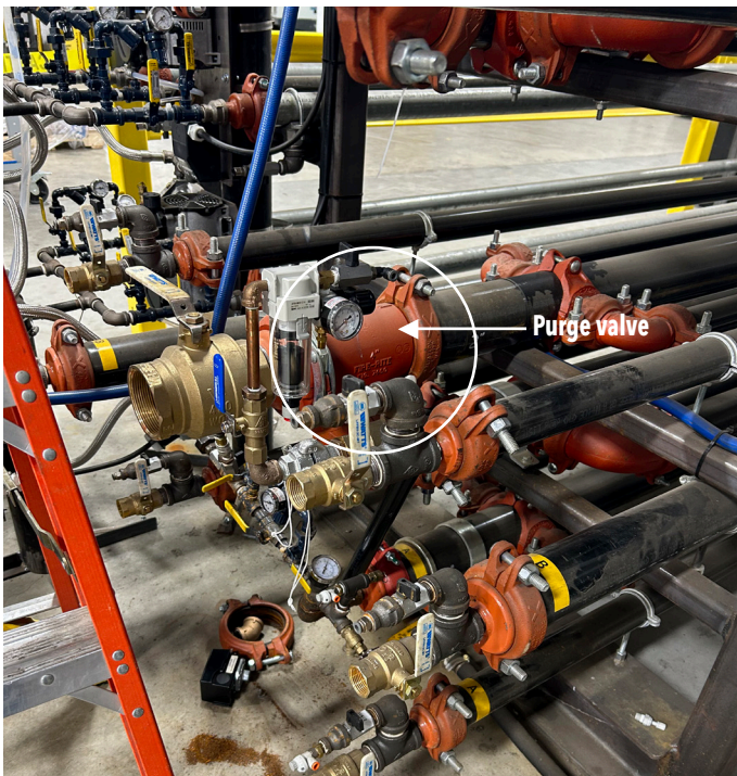
Figure 6. Breathable purge valve for Test 2.
