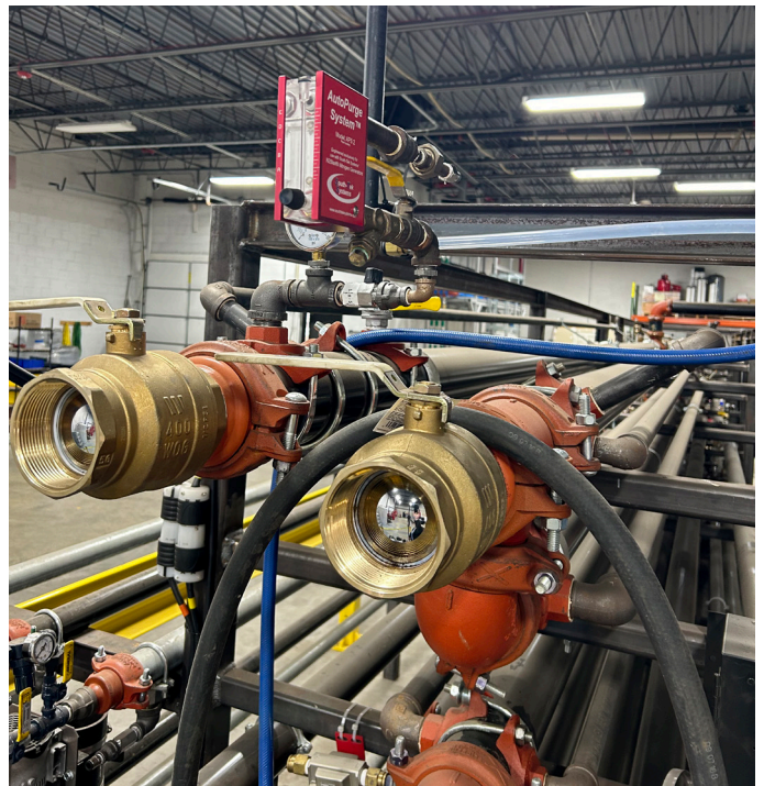
Figure 7. Continuous purge valve for Test 3.
